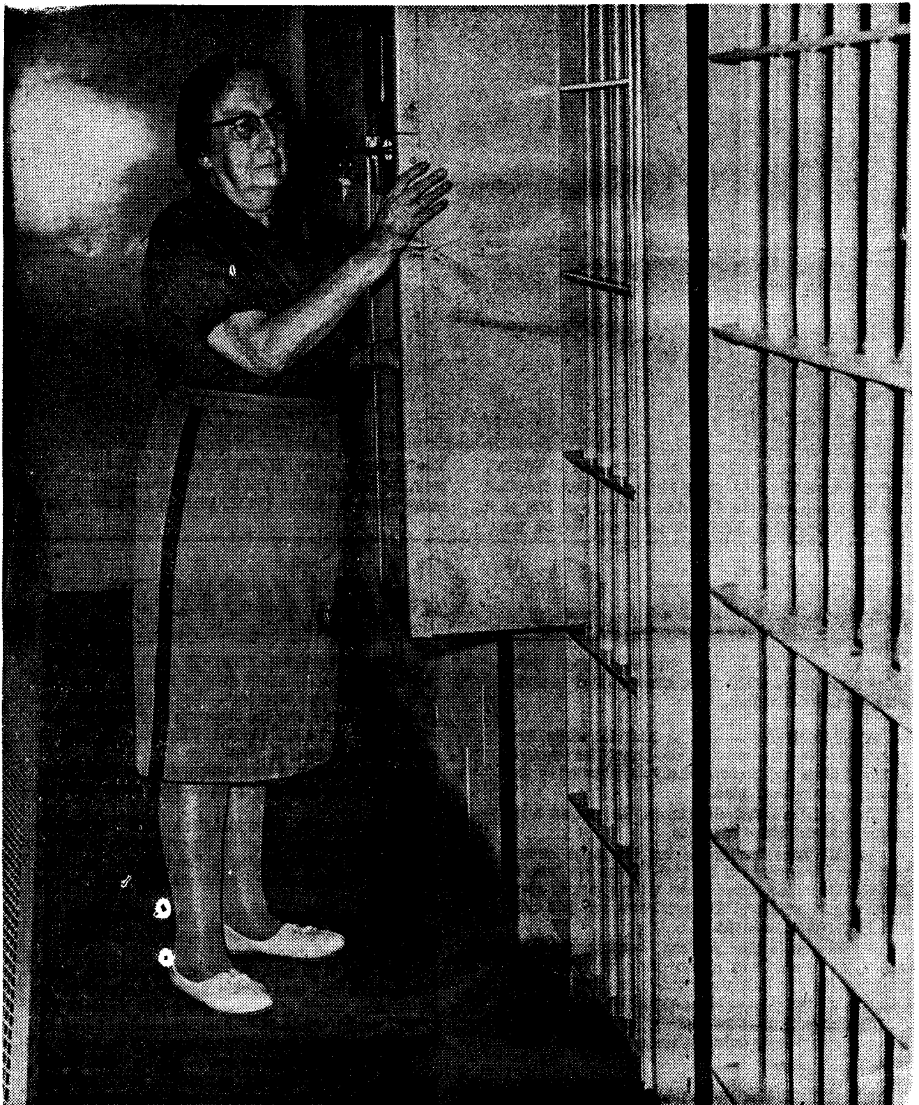
REMOTE CONTROL — Prisoners are locked into their cells, or released, by means of a remote control box, here operated by Mrs. Rita Dagenais. Visitors are not allowed in this area but see detainees in a special room on the first floor of the Cumberland County Jail. (Staff Photos by John A. James)
