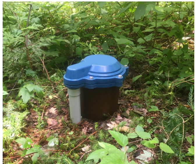
Wellhead with a sanitary seal, Poplar Stream Falls Hut
