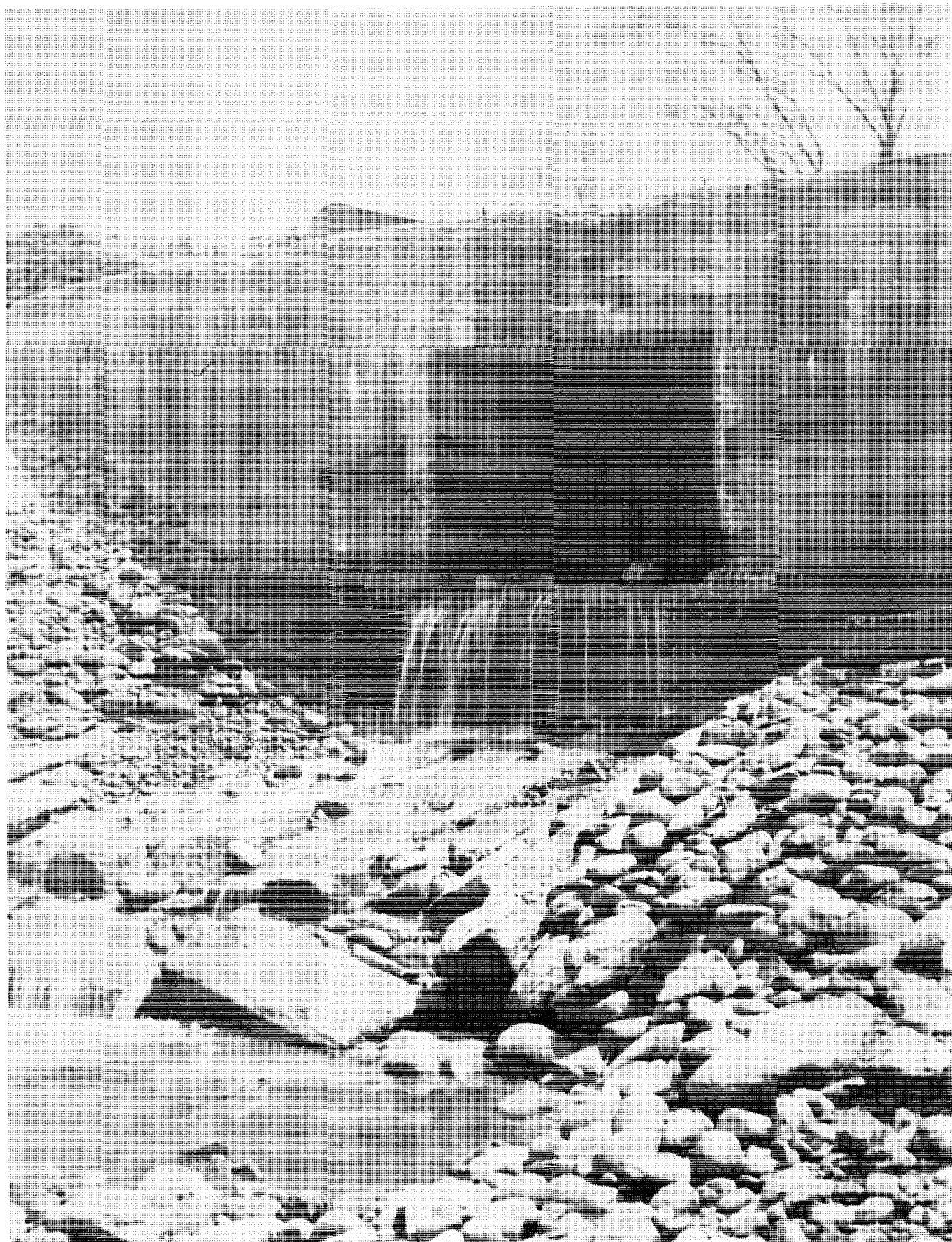
4 x 5 FOOT PUBLIC SANITARY AND STORM SEWER, AT PERIOD OF VERY LOW FLOW, DISCHARGING TO BANK OF PENOBSCOT RIVER.
