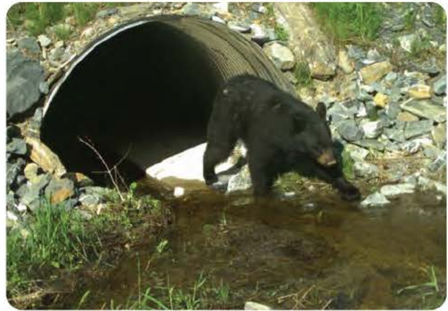
Above is an example of a wildlife habitat connector installed by the Maine Department of Transportation (MaineDOT) as part of the Caribou Bypass (Route 161) Project. Photo by MaineDOT.
