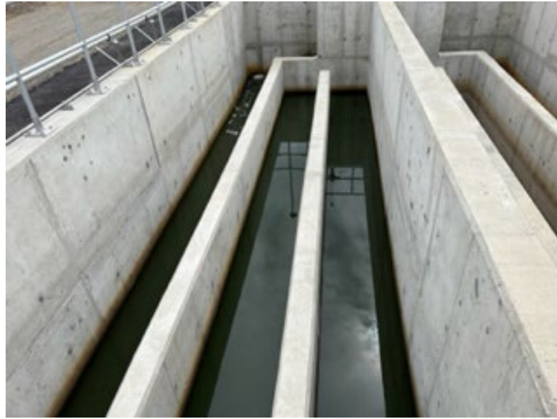
Cl2 Contact Tank
