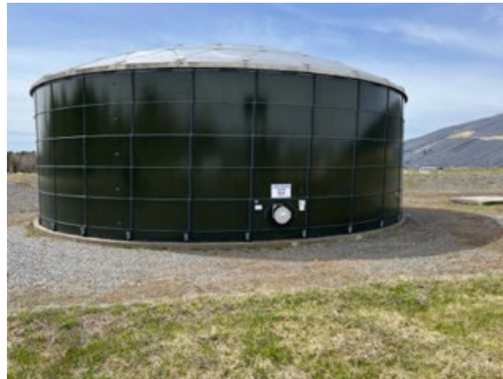
Leachate Storage Tank
