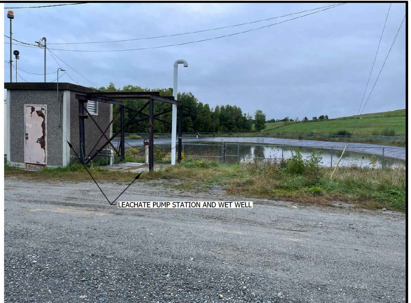
LEACHATE PIPED 3.7 MILES TO TREATMENT PLANT EMWWTP LEACHATE POND AND PUMP STATION
