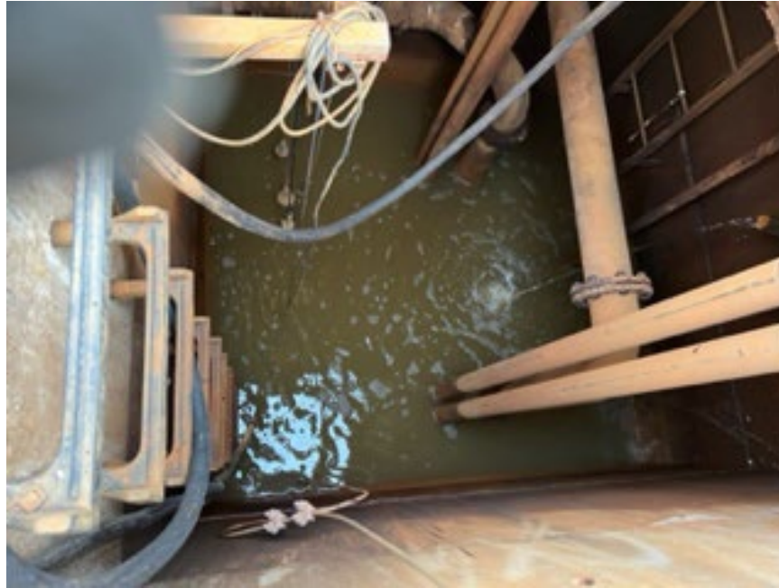
Pumpstation Wet Well
