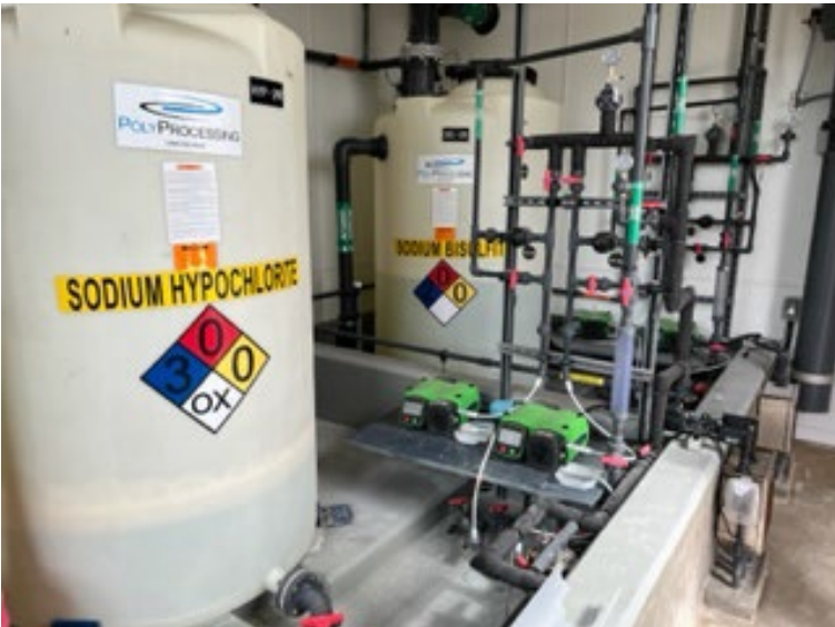
NaHSO3 and NaOCl Tanks
