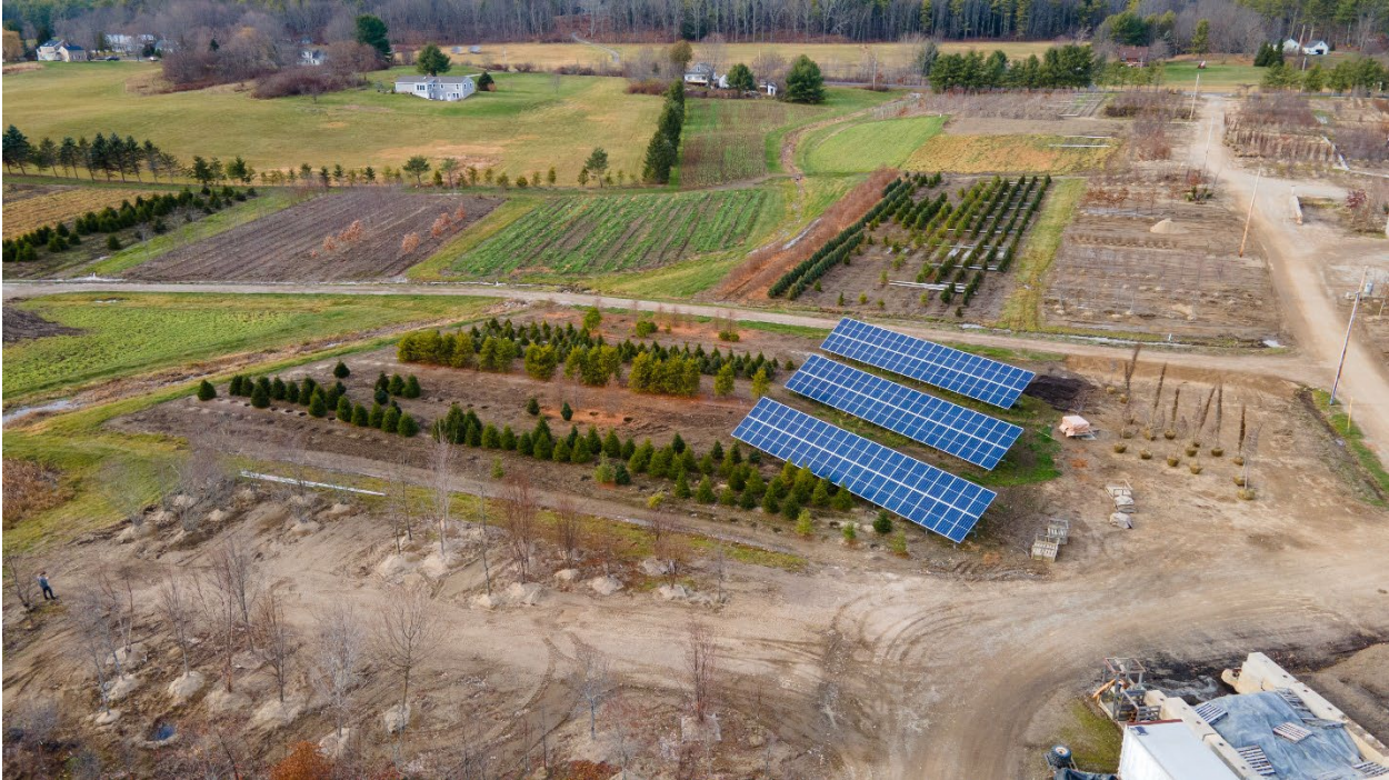
Photo credit: ReVision Energy
