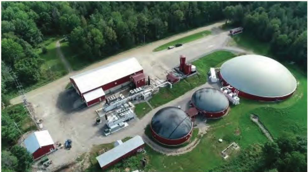
The digester facility at Agri-Energy in Exeter processes food waste to extract methane gas for energy on a continuous 24/7 system.
