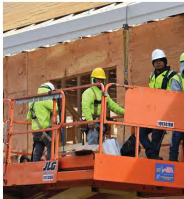
The Snow School Project in Fryeburg is an example of housing retrofits helping to upgrade and expand Maine’s existing housing stock to meet growing demand.
