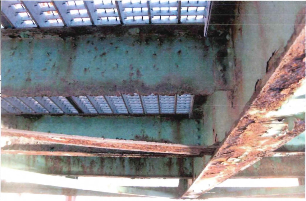
Deck stringer bottom flange separated from web
