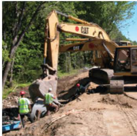
After years of increasing need and congestion, the Kittery-to-South Portland widening project broke ground in 1997.
