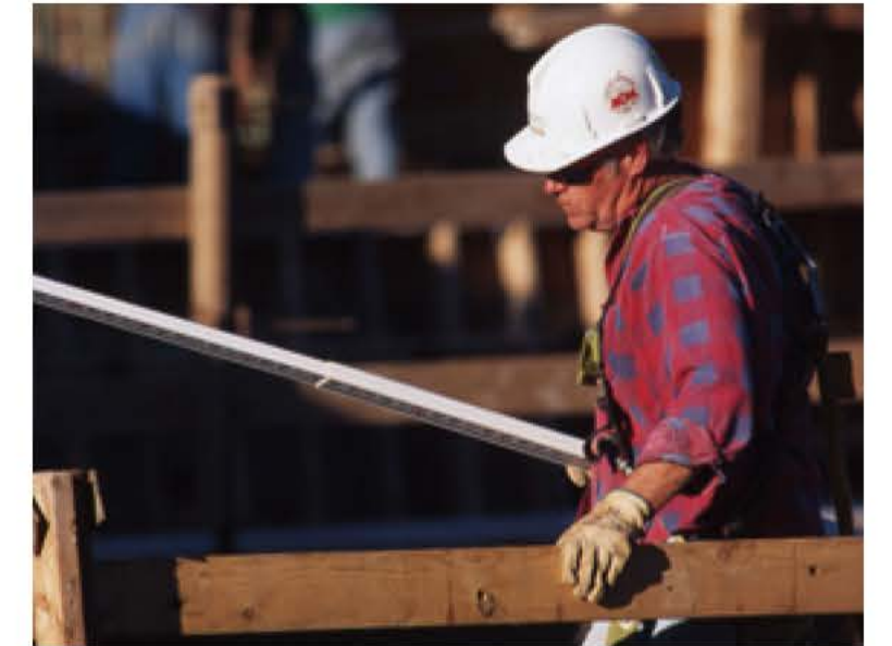
From May of 2000 through 2005, history repeated itself as contractors completed a 30-mile, $135 million renovation of New England's 1947 vintage superhighway.
