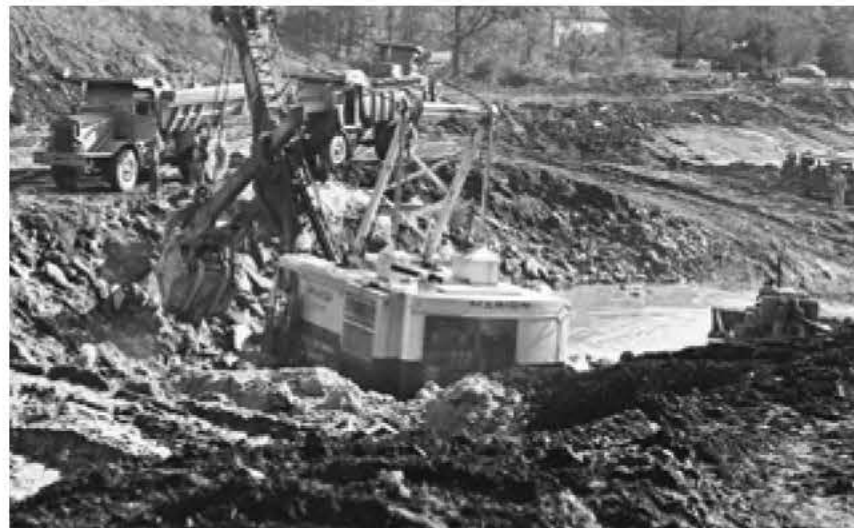
More days than not, epic rainfall, acres of mud, and deep water greeted the construction crews at work on the Turnpike's Portland-Augusta extension.
