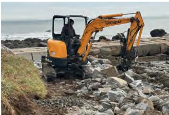
Cleanup crews begin the process of rebuilding the Rockland Harbor Trail where it meets the breakwater following the January storms that damaged the waterfront. (Credit: City of Rockland)
