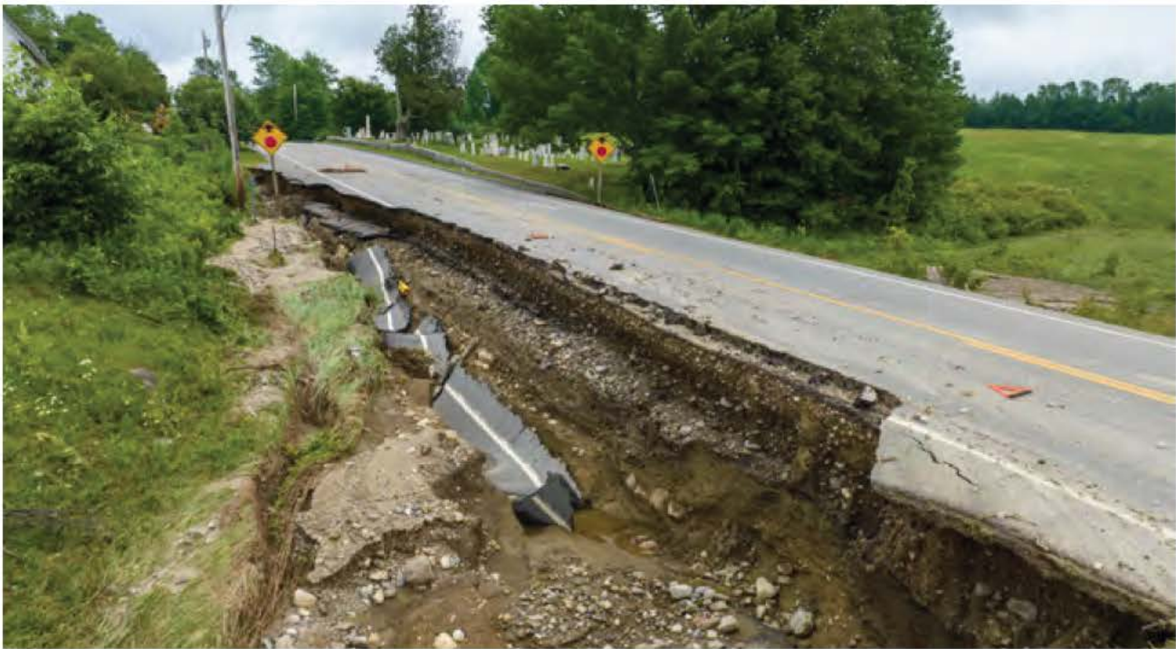
Parts of Route 133 in Jay, Maine sustained heavy damage from runoff during an historic summer rainfall in June 2023 that required months of repairs.
