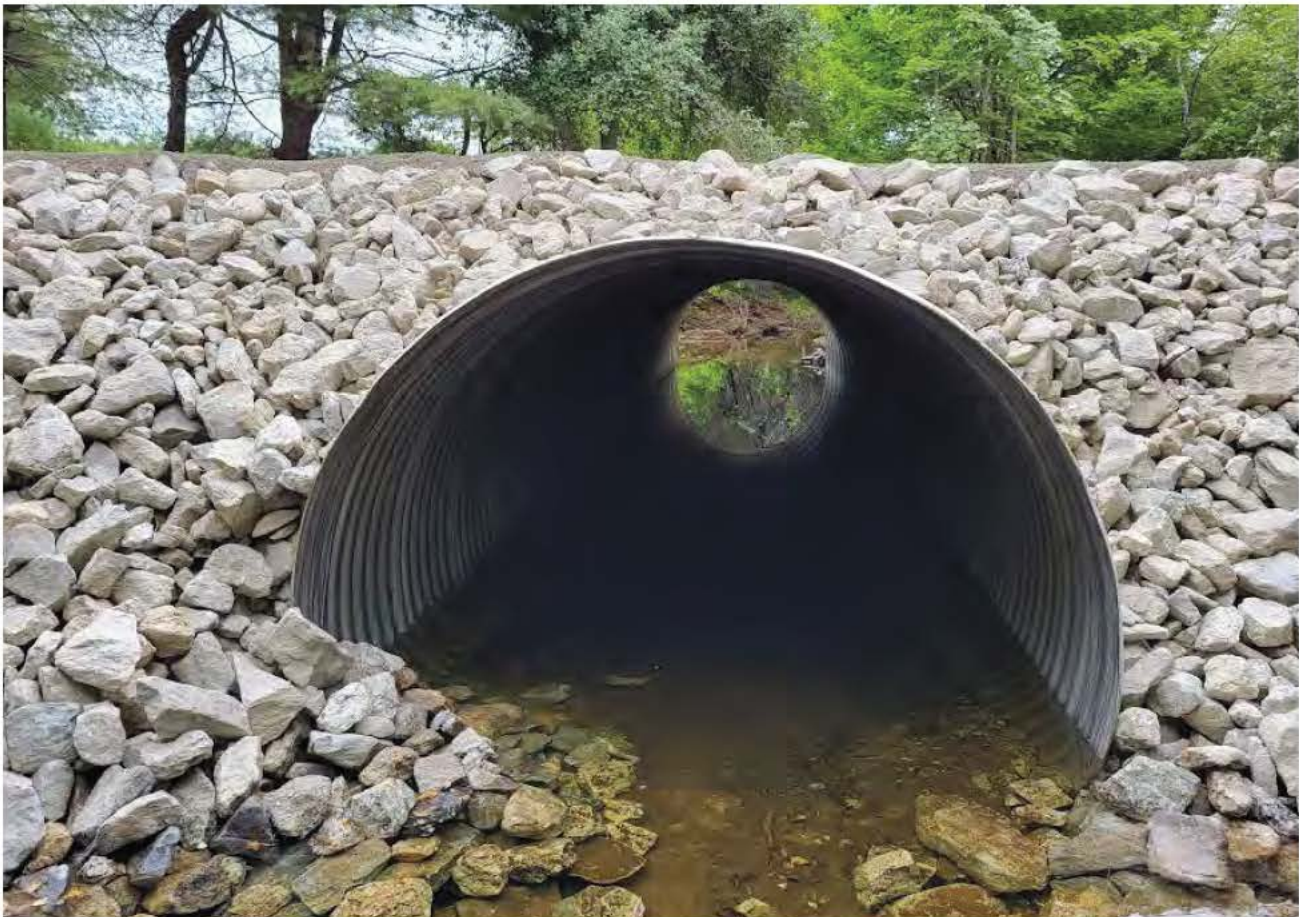
This culvert in Paris, Maine was constructed in 2023 to withstand extreme weather events, and was undamaged during the storms in 2024. Credit: Maine DOT
