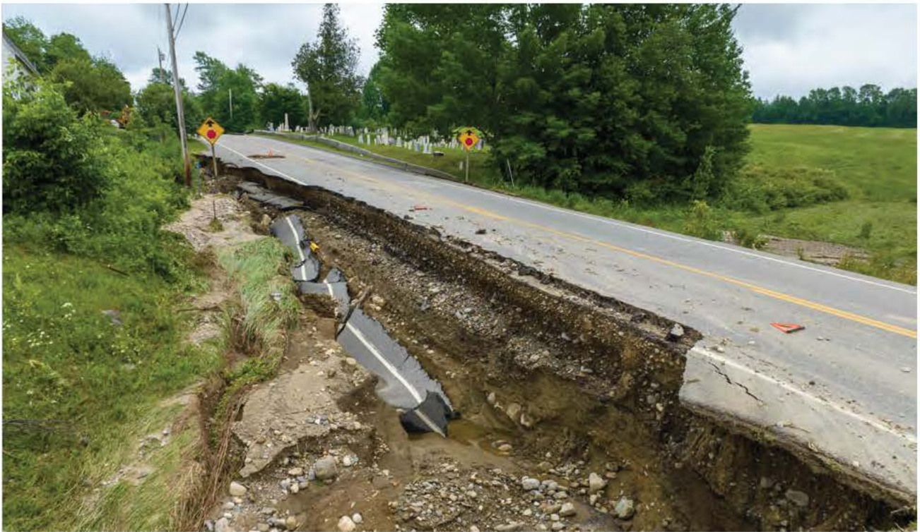
Parts of Route 133 in Jay, Maine sustained heavy damage from runoff during an historic summer rainfall in June 2023 that required months of repairs. Credit: Maine DOT
