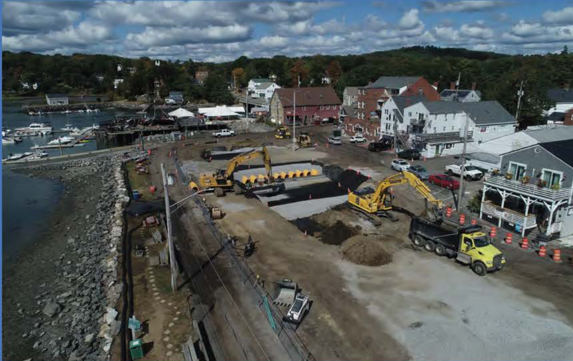
A work crew wraps up installation of the new underground stormwater retention system in Damariscotta last September. Credit: Town of Damariscotta
