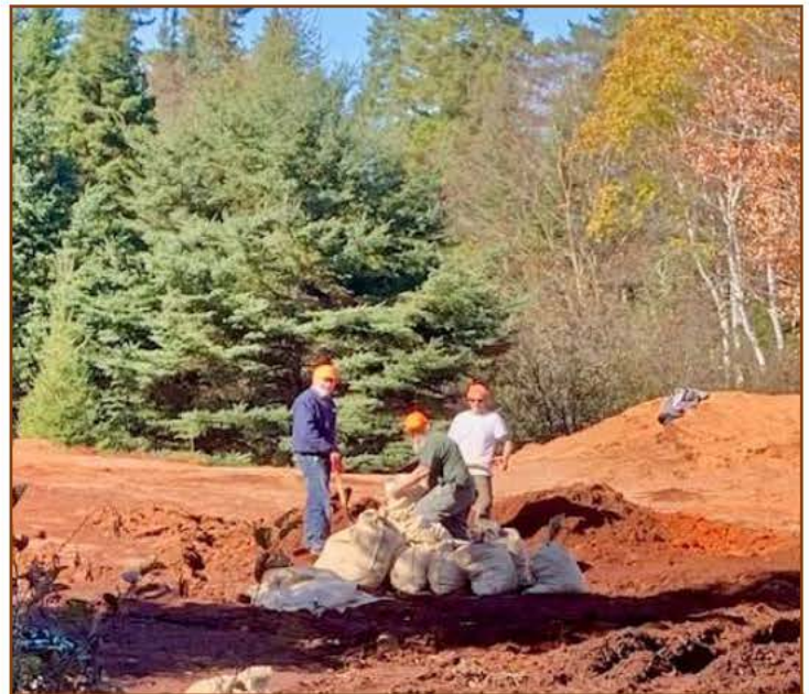
Rangers and volunteers filling burlap bags for leakage mitigation efforts at Telos Dam.
