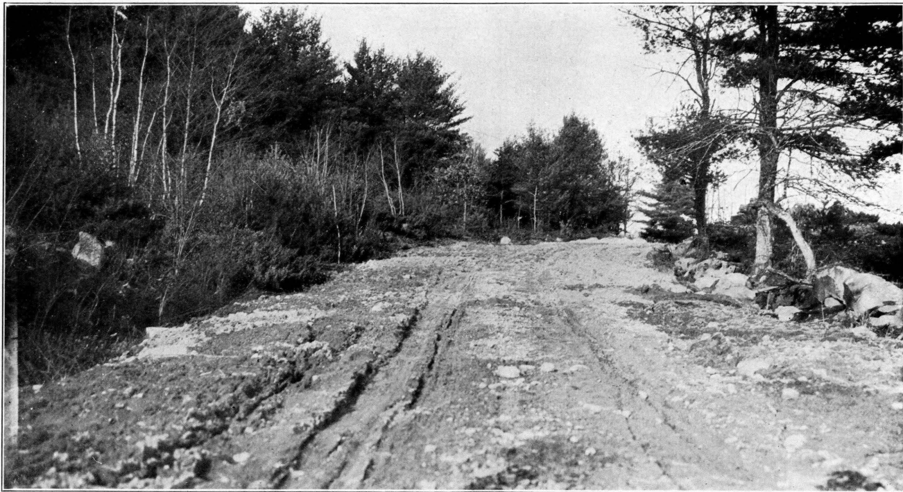
Kennebunkport Trunk Line before improvement.
