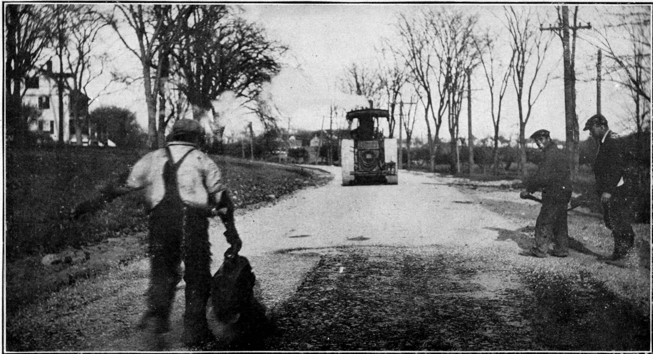
Federal Aid Road. Showing second application, one-half gallon of hot asphaltic oil completely filling voids; immediately followed by a covering of stone screenings and then rolled.
