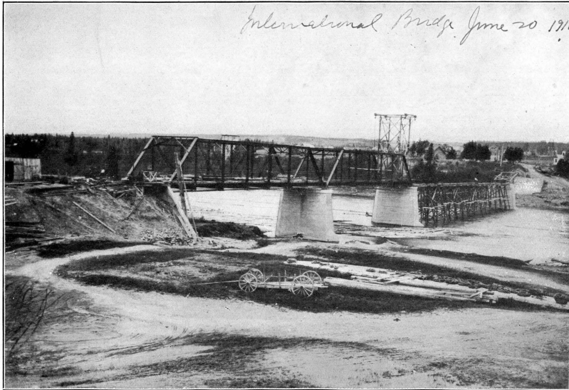
International Bridge between Van Buren, Maine and St. Leonards, New Brunswick. In process of erection. June, 1911.
