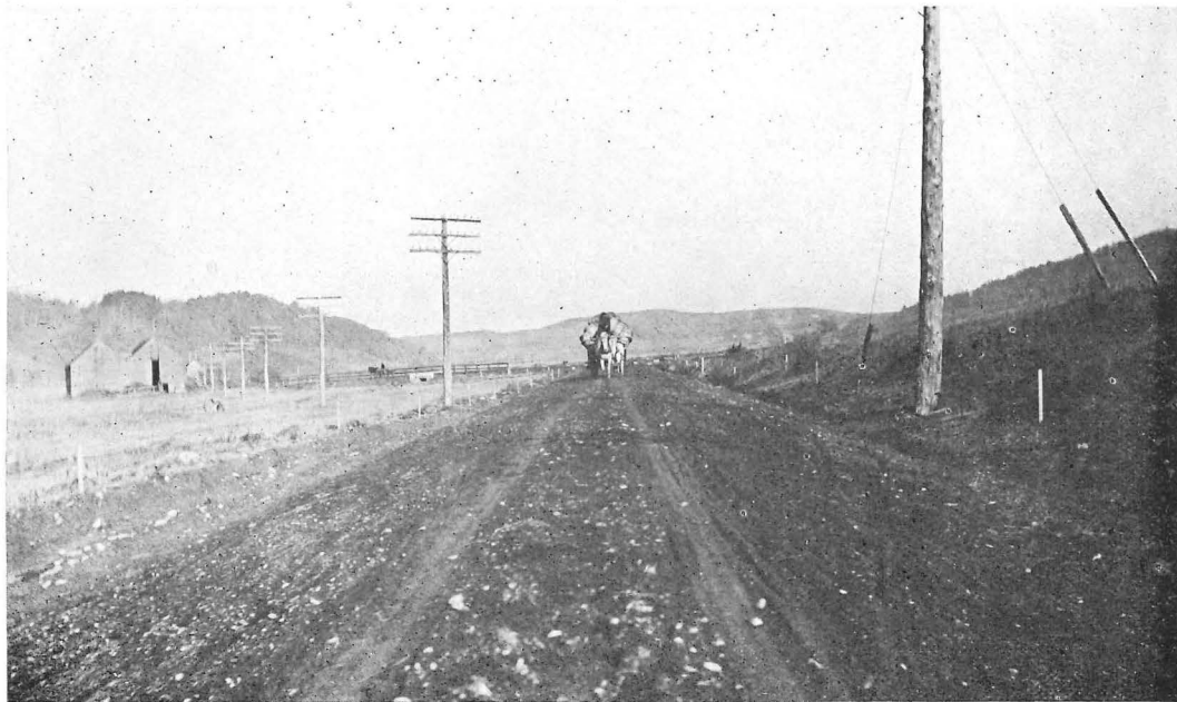
Rockland. 1908 section. Finished road. Eight inches of selected gravel placed in two courses over Telford base. Contract let to city. T. E. McNamara, Commissioner
