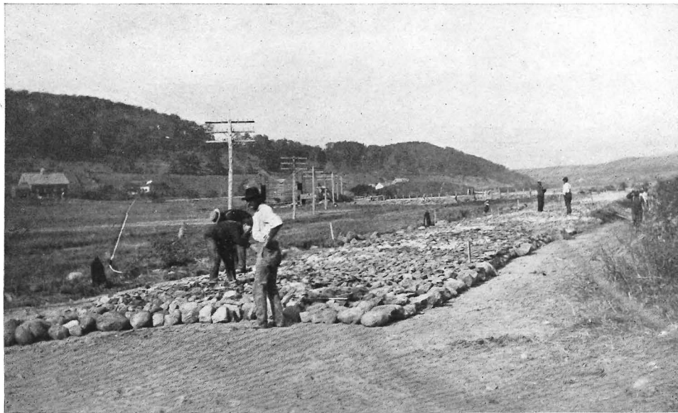
Rockland. 1908 section. Telford base. Workmen sledging stone chips to bind base. Contract let to city. T. E. McNamara, Commissioner
