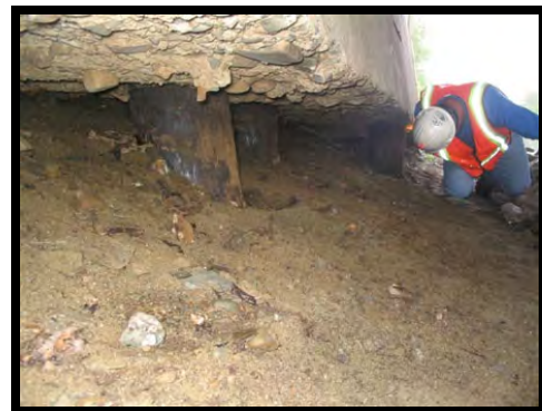
Abutment scour with exposed timber piles
