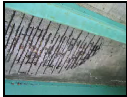
Concrete spalling and exposed reinforcing steel
