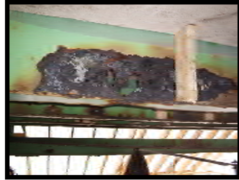
Advanced corrosion and section loss
