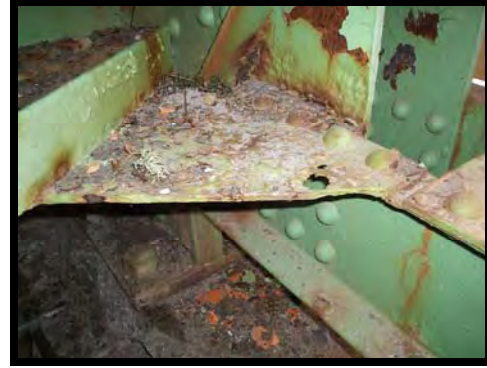
Corrosion of a structural connection
