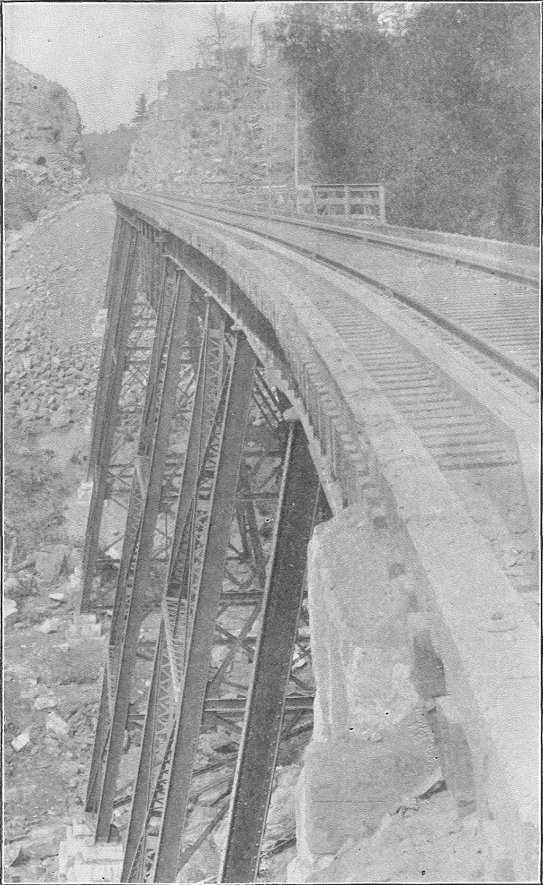
NEW VIADUCT AT BUNKER BROOK, SHOWING CUT IN CHANGED LINE. Bangor and Aroostook Railroad.
