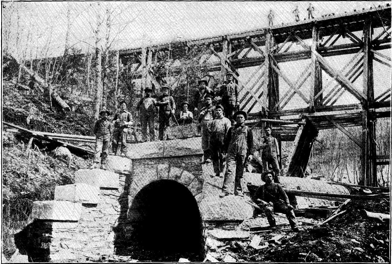
CULVERT MASONRY, UNDER AN OLD TRESTLE, NOW FILLED. Bangor and Aroostook Railroad.
